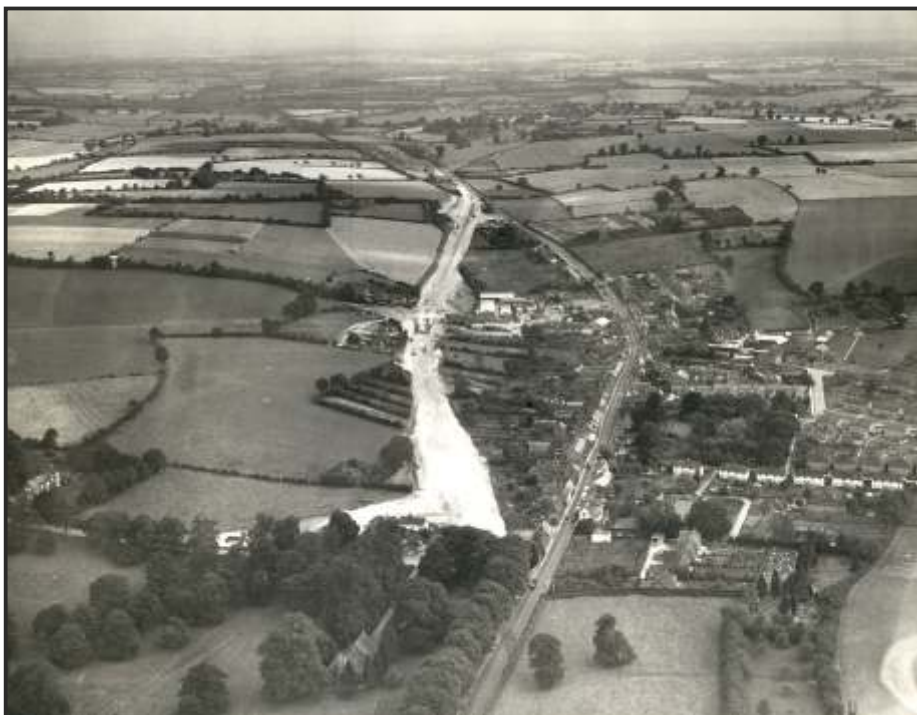
Construction of the Markyate bypass in 1955 showing the chalk revealed by removal of topsoil, aerial view looking south (BEAMS photographic archive)
