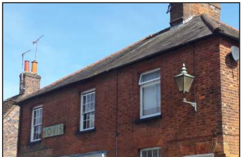
Replacement window on right side at first floor level is at odds with the original sash windows to the front elevation of 73 and 75 High Street
